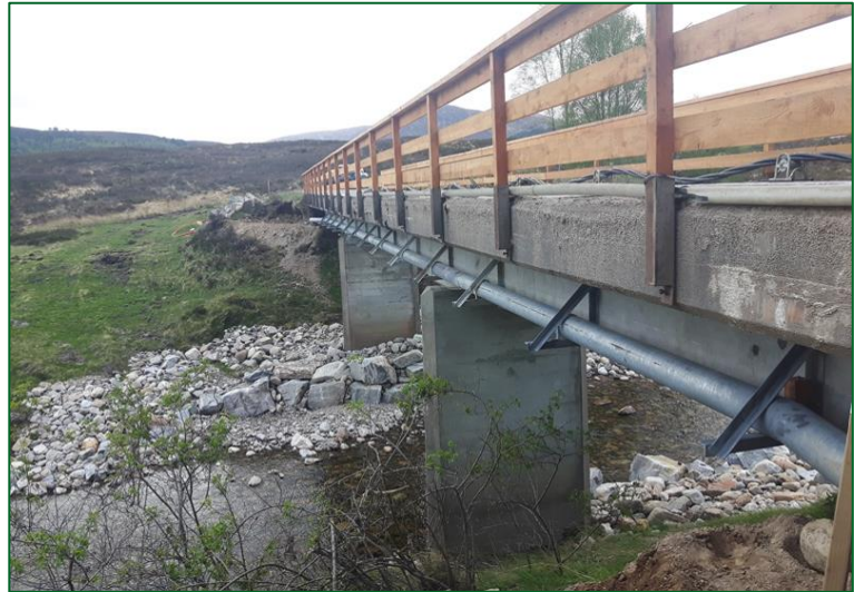
Electrical cables laid across Chisholm Bridge in a steel duct
