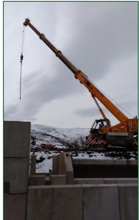
Allt Garbh – Precast units all installed, despite the weather. Top marks to the crane operator and Sinclairs in getting a 60 tonne crane into this location.
