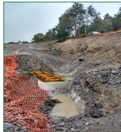
Abhainn Gleann nam Fiadh – powerhouse excavation complete. Blinding and rebar placed for turbine sump (right).
