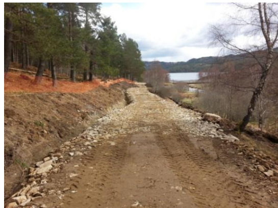
The existing access track from Chisholm Bridge (public road) to the powerhouse has been widened for construction access
